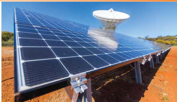
ESA's deep-space ground station at New Norcia, Western Australia, is now powered in part by sunlight, from a new solar power 'farm' completed in August 2017. The farm has 840 photovoltaic panels arranged in five double rows with a rated capacity of 250 kW. Source: https://commons.wikimedia.org/wiki/File:New_Norcia_solar_ESA387214.jpg
